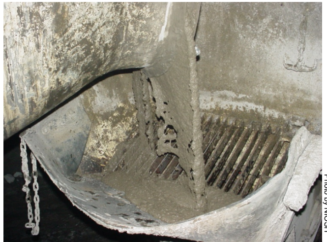
Figure 31. Consistency of wet mix shotcrete being loaded into the hopper of a shotcrete machine.
