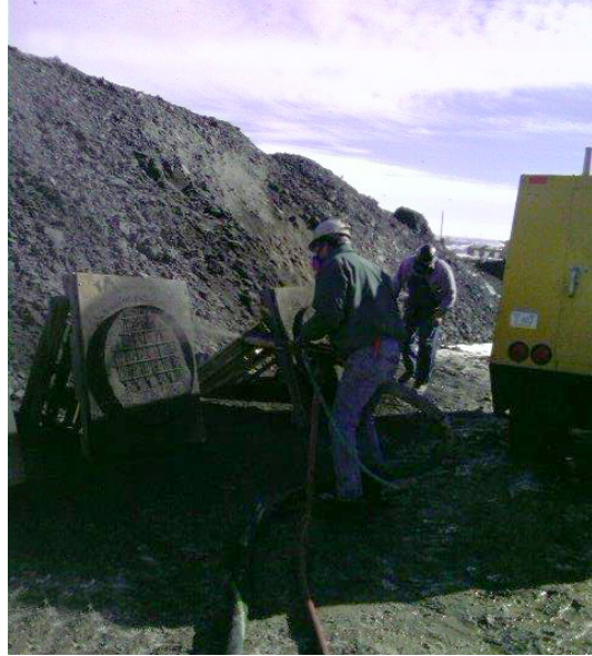
Figure 96. Shooting wet mix shotcrete into a round panel form with wire mesh reinforcement.
