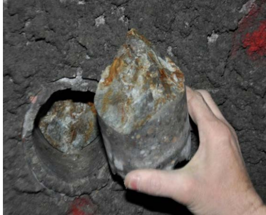
Figure 69. Adhesion test #3: drill hole and core indicating a tensile failure located primarily in the host rock.
