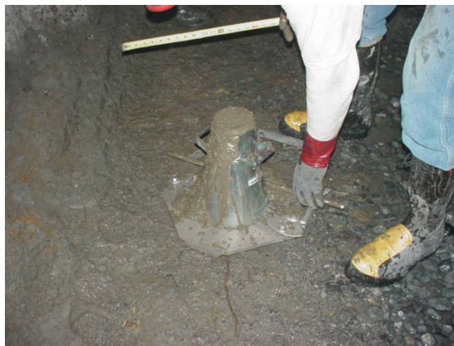
Figure 32. Filling a slump cone with wet mix shotcrete prior to conducting a slump test in an underground mine.
