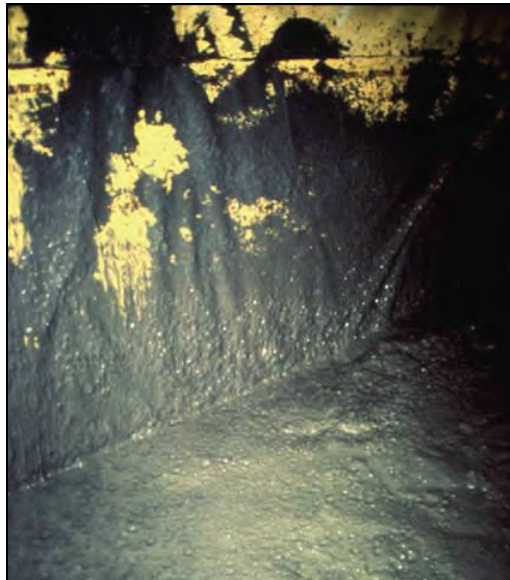
Figure 25.—Inside the formwork of a typical pumpable seal showing the brattice liner and the cementitious filling material.
