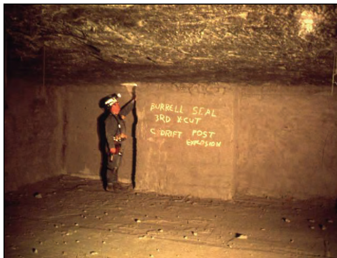
Figure 47.—Completed 24-in-thick Omega block seal showing the angle iron hitch along the ribs and floor and the outer surface coated with an approved sealant.
