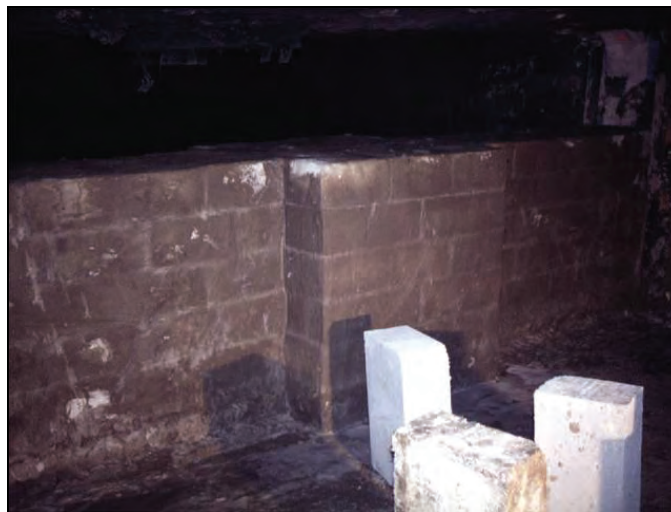
Figure 45.—Construction of a 24-in-thick Omega block seal with hitching and a center pilaster. All surfaces are coated with BlocBond mortar.
