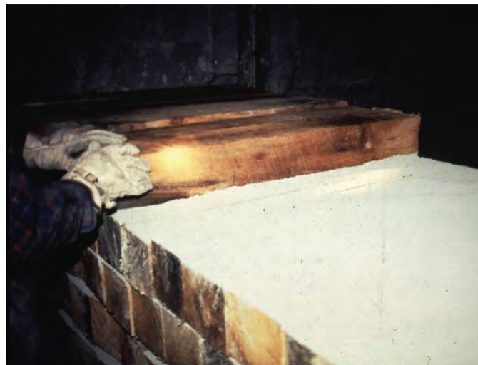
Figure 39.—Closeup of a hitched wood-crib-block seal showing the layer of rock dust placed between each layer of wood crib blocks.
