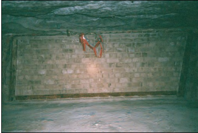
Figure 29.—Completed solid-concrete-block seal without a center pilaster showing the angle iron hitch on the ribs and floor only.
