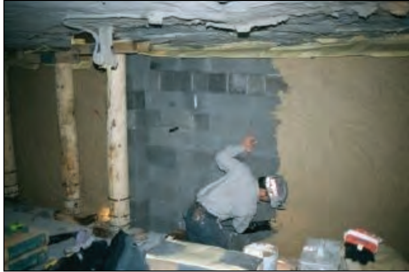
Figure 31.—Tongue-and-groove, solid-concrete-block seal with center pilaster using pressurized Packsetter grout bags in lieu of hitching around the seal perimeter. The worker is coating the seal with an approved sealant.
