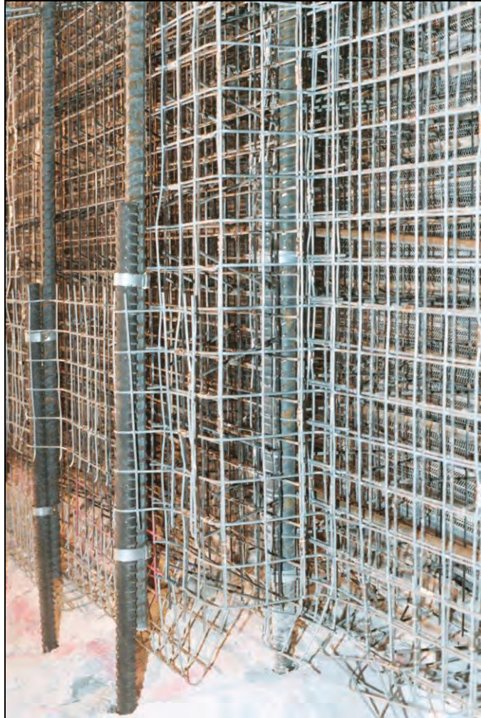
Figure 19.— Insteel 3-D seal under construction with the addition of the front Insteel panel and the front plane of vertical #8 steel reinforcement bars.
