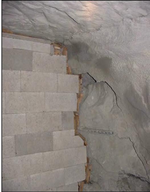
Figure 33.—Dry-stacked concrete block stopping showing wedges used to fit the stopping to ribs and small cut blocks and a wood plank at the top.
