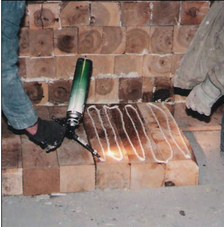
Figure 42.—Construction of a wood-crib-block seal with pressurized Packsetter grout bags in lieu of hitching showing the application of glue between all wood-crib-block surfaces.
