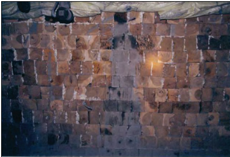
Figure 43.—Construction of a wood-crib-block seal with pressurized Packsetter grout bags in lieu of hitching showing the glued wood crib blocks and the grout bags used along the roof and ribs. The active-mine-side surface is later covered with brattice and coated with an approved sealant.
