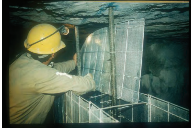
Figure 21.—Closeup of Meshblock seal under construction showing the Meshblocks and the vertical #8 steel reinforcement bars and anchors.
