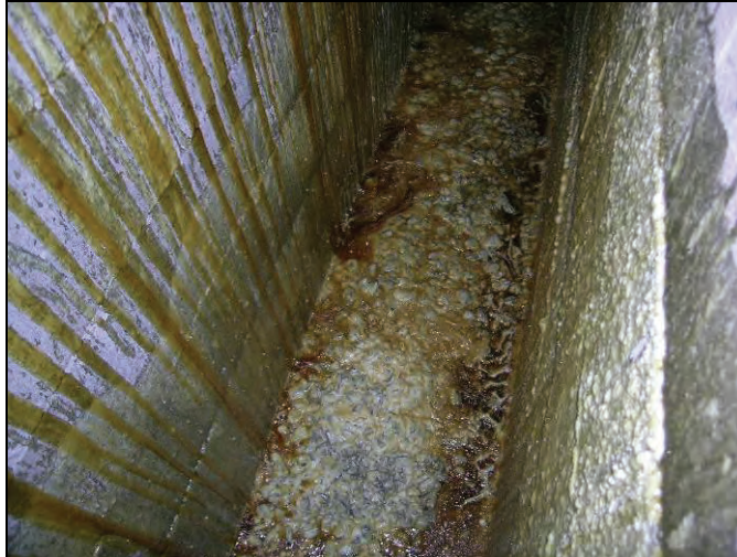
Figure 37.— Polymer and aggregate seal from MICON showing the rear and front form wall, the polymer coating on the inner surfaces of the form walls, and the polyurethane foam and aggregate mixture filling the inner core of the seal.
