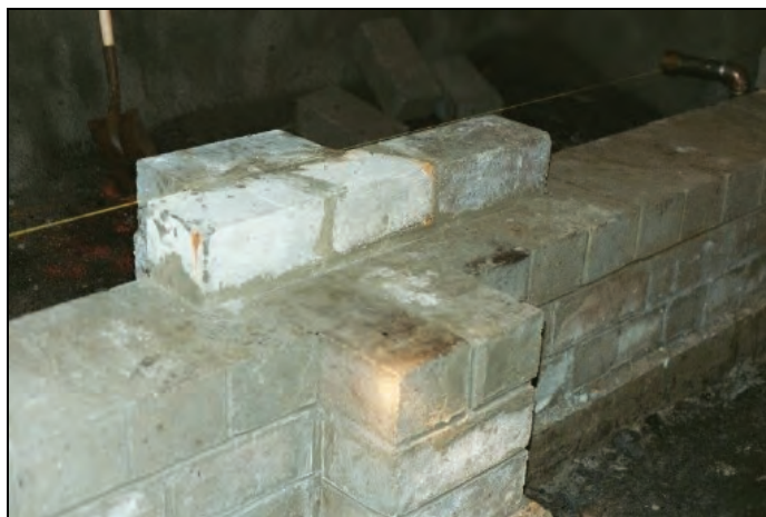
Figure 27.—Solid-concrete-block seal under construction showing the center pilaster and the fully mortared joints on all sides.
