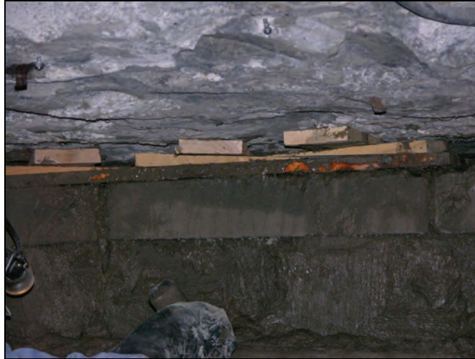
Figure 46.—Construction of an Omega block seal showing the wood board and wedges used to secure the seal at the roof.
