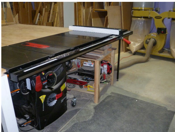
Figure B1. Woodshop table saw with exhaust duct connected to the dust collector. Photo by NIOSH.
