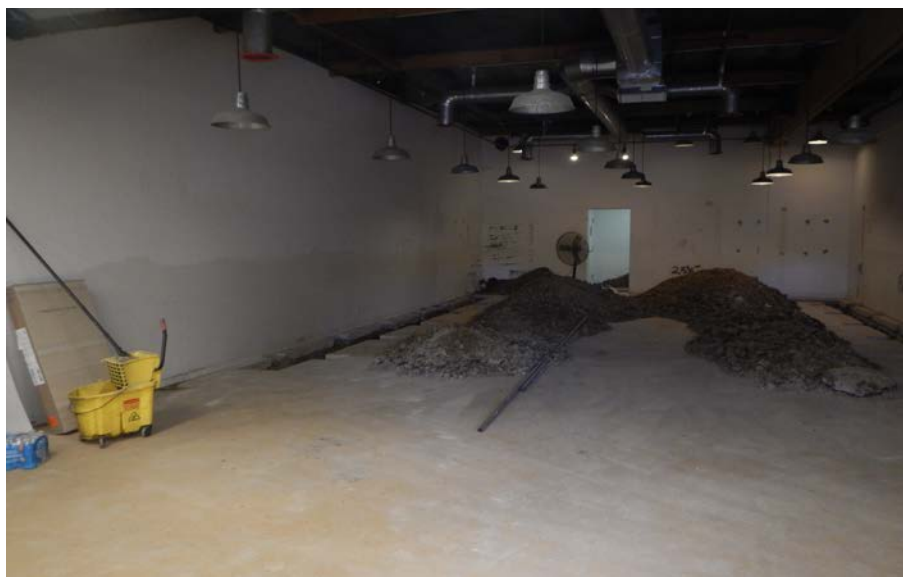
Exhibit 2: The rear left corner of the store space where the victim died. Note: The trenches were dug after the fatality.
