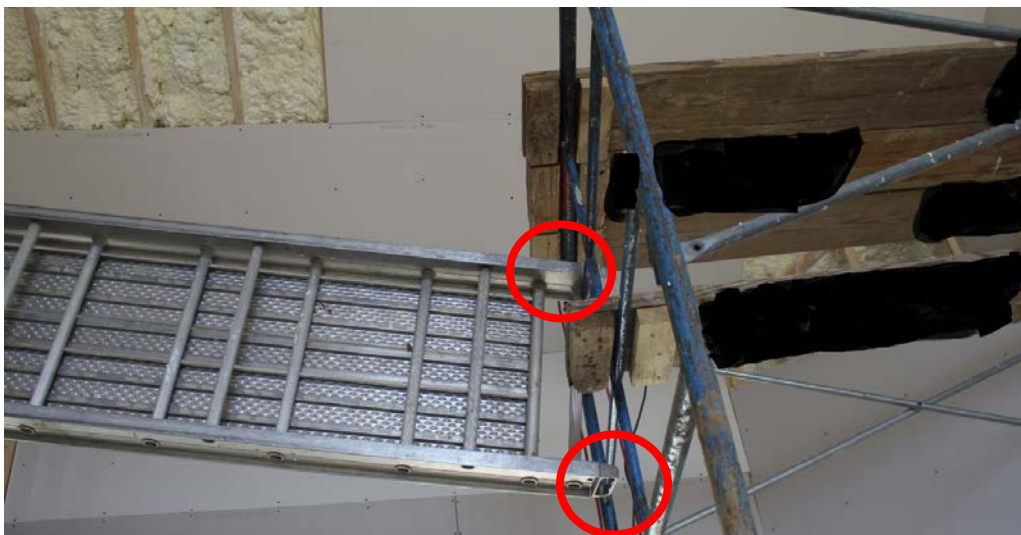
Figure 3. Position of the plank after the accident. Note the lack of attaching hooks (circled)
