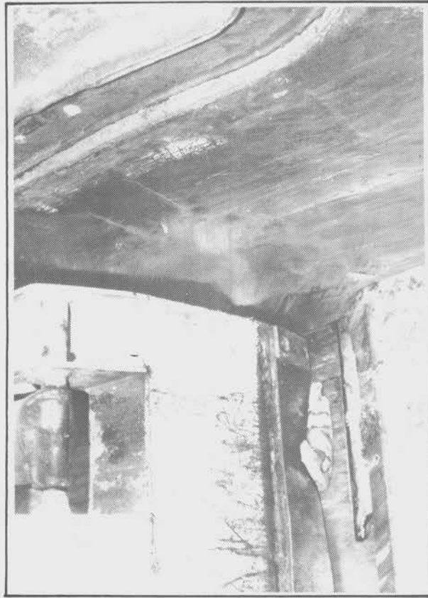
Figure 74. Panel-to-side-wall shear point.
